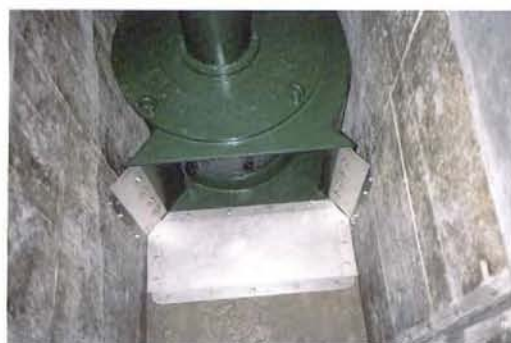
PUMPING STATION 25RM
